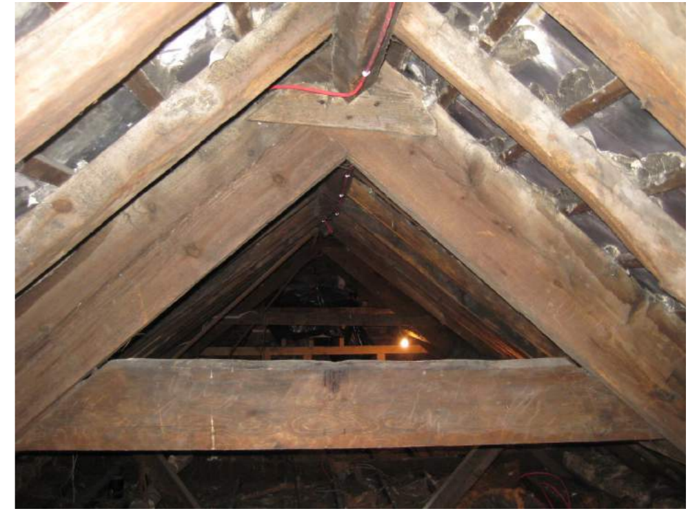
DETAILED VIEW OF THE ROOF STRUCTURE SHOWING THE DISINTEGRATED MORTAR BED TO THE UNDERSIDE OF THE SLATES
